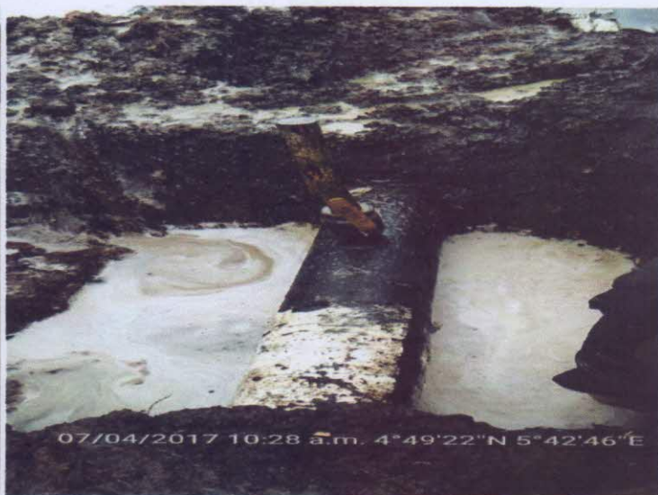
B: LEAK POINT AFTER OPENING AND PEGGING
