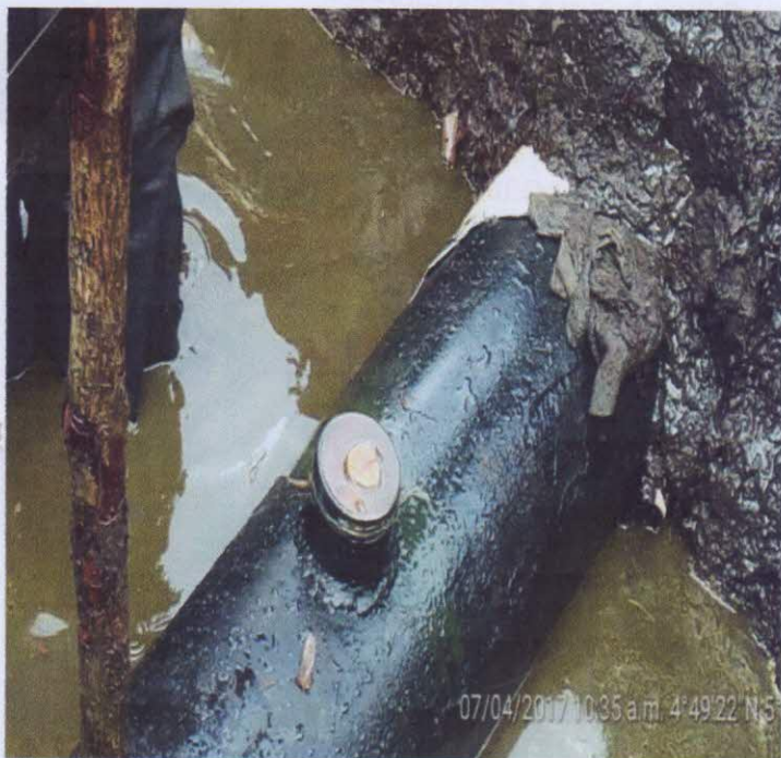
C: CONING OF LEAK POINT
